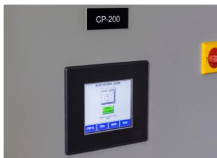
Control panel interface
